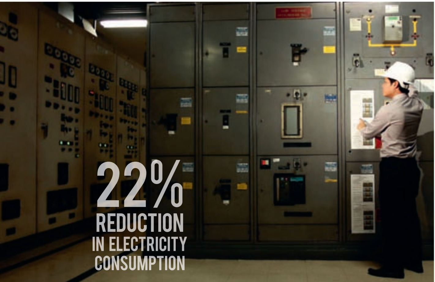
Equipment room at Tower One & Exchange Plaza, Makati City
